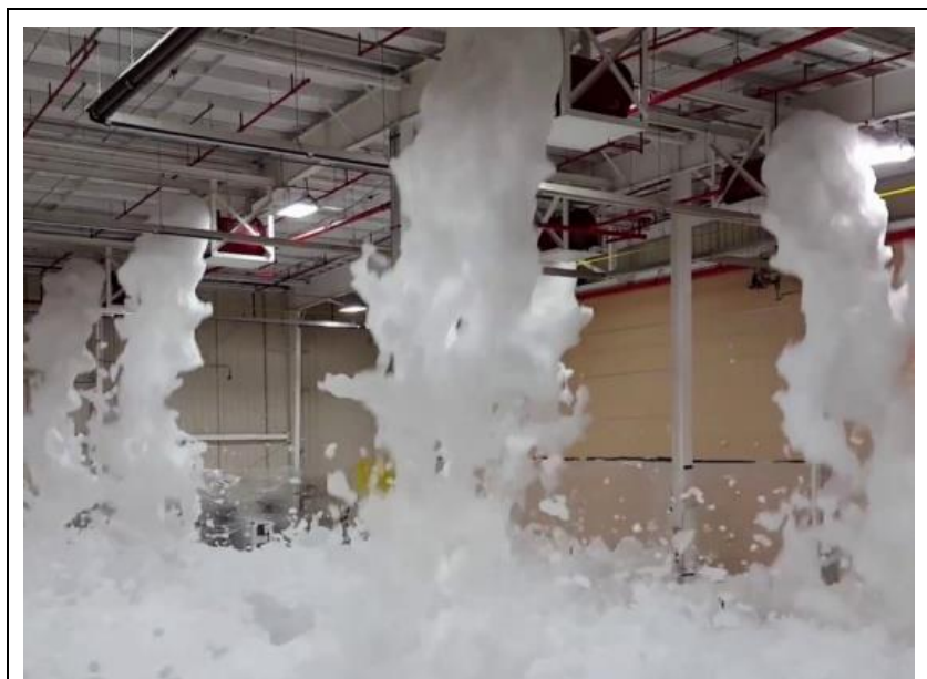
High expansion foam system operation in a warehouse
