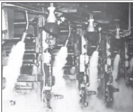
A CO 2 Extinguishing System that has been activated
